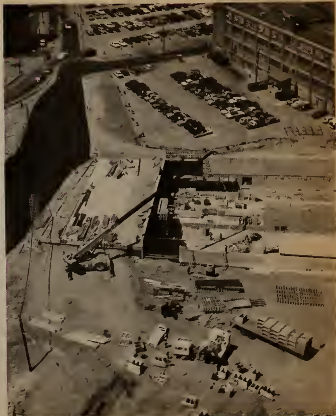
Ruggles Street Station area showing station platform area and new Ruggles Street under construction.
